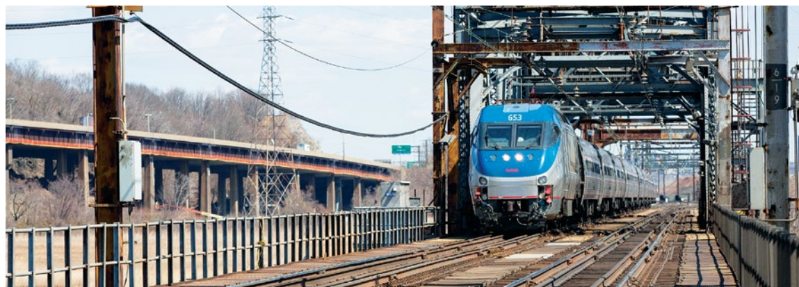
The 108-year-old Portal Bridge just outside Secaucus, N.J., has long been a major bottleneck on Amtrak's Northeast Corridor. The busiest train span in the Western Hemisphere, it carries nearly 200,000 passengers per day across the Hackensack River, but speeds are limited to 60 miles per hour due to its deteriorating condition. Photos courtesy of Amtrak
